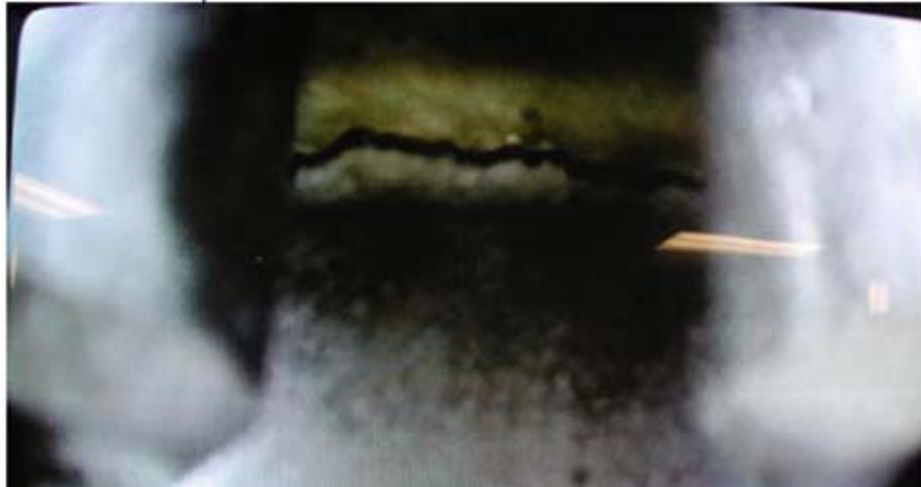
Figure 4.3: Crack at the Top Flange Neck of a Tapered Stress Joint (Confidential Source)
