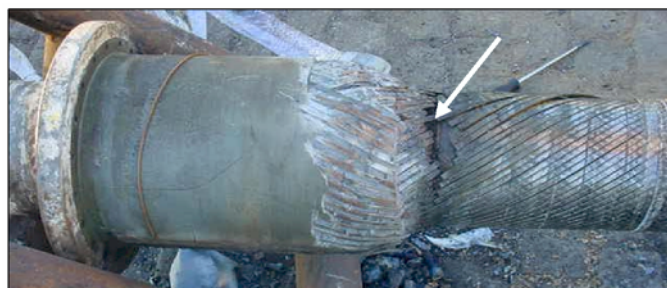
Figure 4.6: Tensile Armor Wire Failure at End Fitting [Ref. 22]
