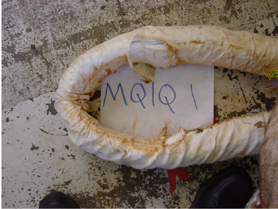
Figure 8.9 MQIQ 1 Wear of Outer Cover at Point Where Rope First Makes Contact with Spool (Tangent Point)
