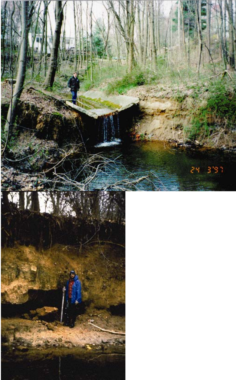
Figure 12: Examples of severe undercutting of stream channels.
