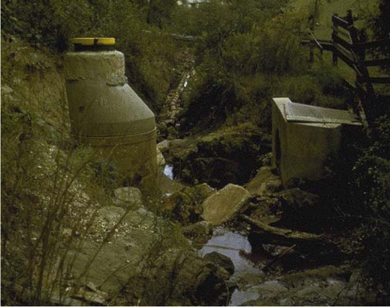
Figure 11: Severe down-cutting of stream channel has exposed utility features.
