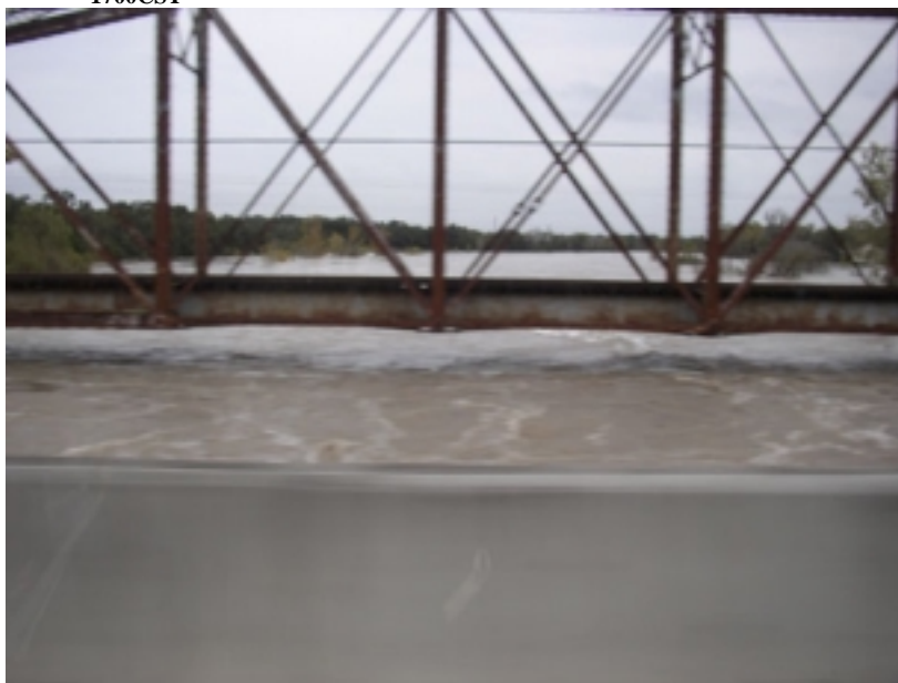
Flash flood wave along Coleta Creek at the Highway 59 bridge. See episode narrative below for additional details and rainfall totals.
