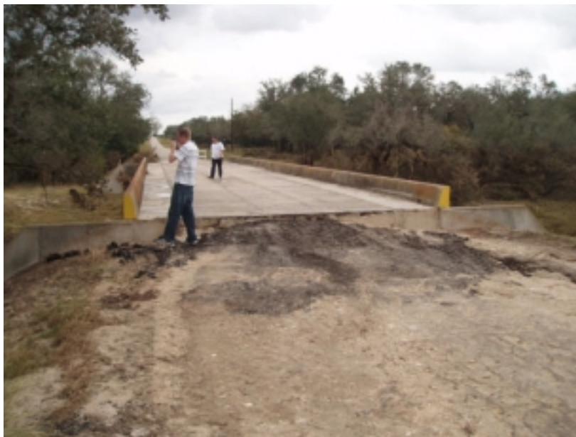
Washed out roadway from flash flood of Perdido Creek. Further up this road a bridge was completely washed out from Perdido Creek. See episode narrative below for additional details and rainfall totals.
