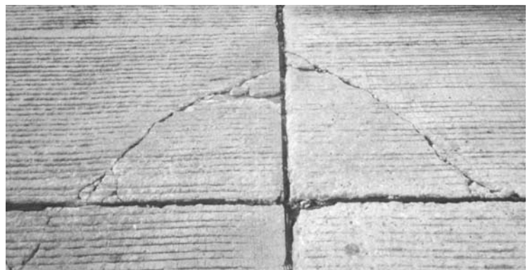
Corner cracking with slight spalling.
