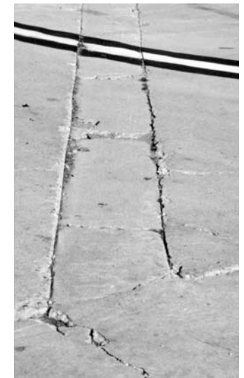
▲ Concrete patch in poor condition.
