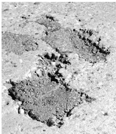
◀ Small surface spall that has been patched.
