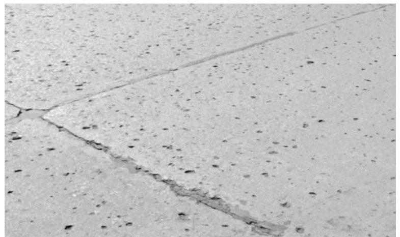
► Extensive pop-outs of large aggregate from surface.
