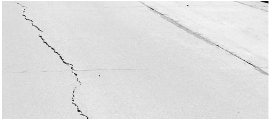
▲ Settlement caused meander crack with faulting.
