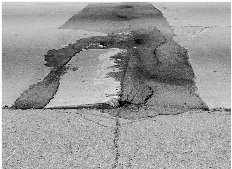
▲ Internal pressure has partially raised slab at the joint. Complete replacement is required.
