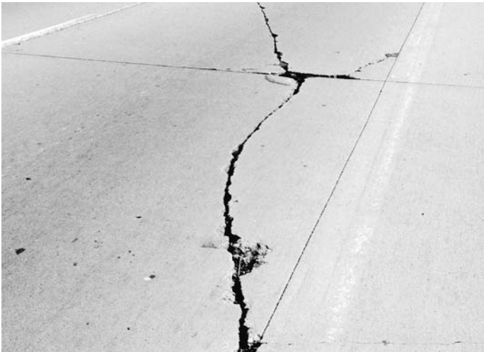
◀ Meander crack caused by settlement. Lack of maintenance allows water to intrude and debris to collect in crack.
