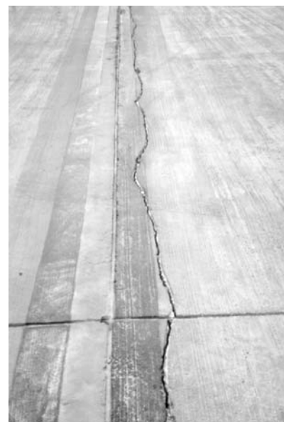
◀ Crack parallel to joint. Open 1/4". No spalling.
