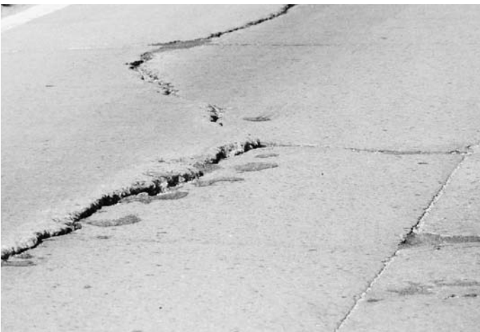
◀ Faulting and spalling of a meander crack.
