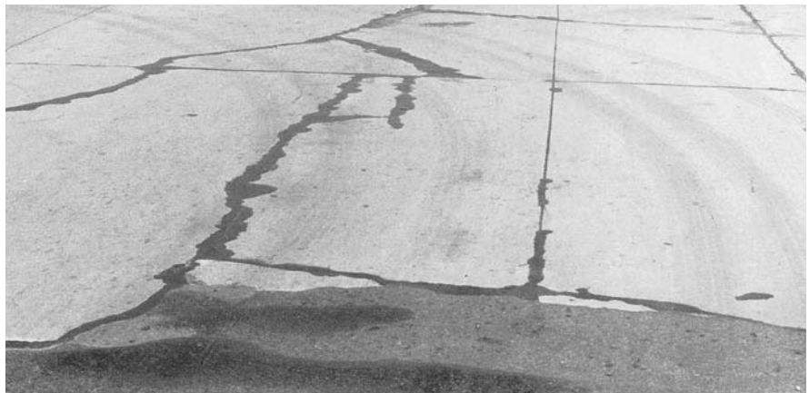
▼ Extensive cracking and patching caused by settlement. Pavement was built on unstable sub-grade soils.
