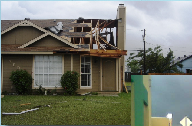
Above: Tornado damage to a home in Killeen. Courtesy of KXXV-TV.
