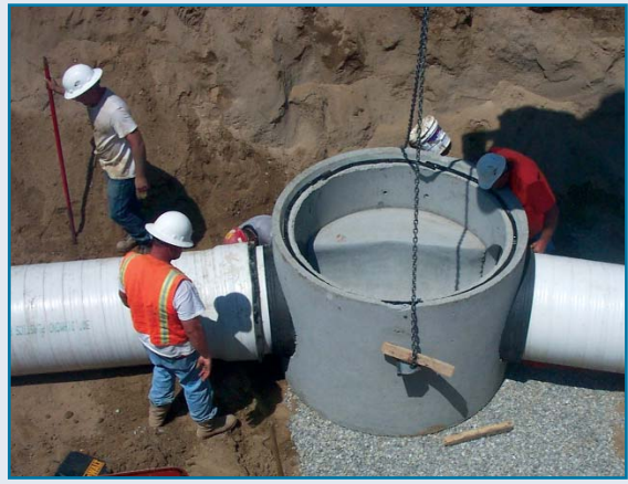
The City of Shafter has worked hard to diversify its primarily agricultural employment base. EDA provided assistance to construct 17,000 linear feet of 30-inch truck sewer collection lines to connect two major industrial areas with a new regional treatment plant. This investment allowed for development of the two new industrial areas on locations outside of the old town site. Completed in October of 2003, it is estimated that this investment will generated 340 new jobs in the near future. It is anticipated that over the next six years the two sites have the potential to create 2,000 jobs and leverage $35 million in private sector funds.
