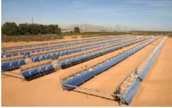
Figure F2 APS Saguaro Solar Trough Power Plant Courtesy of Arizona Public Service (APS)
