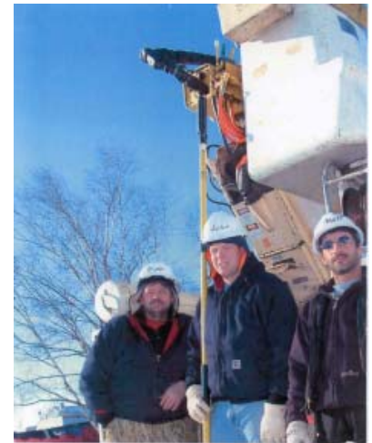
PCB transformer phase-out (Grand Marais, MN)
