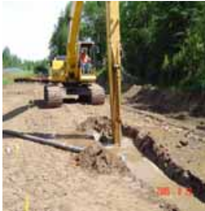
The biopolymer slurry is pumped via a hose into the trench during excavation.
