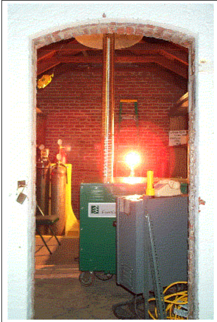
Figure 6. The fuel cell and 1000 watt lamp in the oil building.
