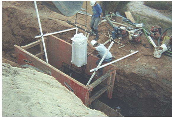
Figure 3. Placement of reactive material into the gate structure of the bone-char phosphate barrier at Fry Canyon, Utah, during September 1997.
