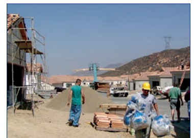
Coordination between the trades on a community scale encouraged quality installations, speedy schedules, and reduced labor costs.
