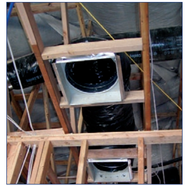
Jump ducts help to equalize a house’s air pressure to ensure air quality and comfort, and provide return air for heating and cooling.
