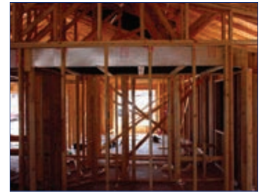
Carefully designed duct runs, placed in interior spaces, save energy and help maintain comfort.
