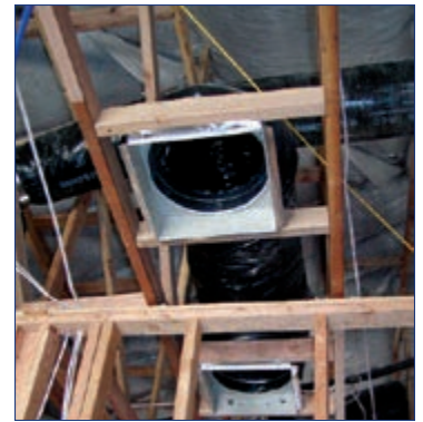
Jump ducts help to equalize a house’s air pressure to ensure air quality and comfort, and provide return air for heating and cooling.
