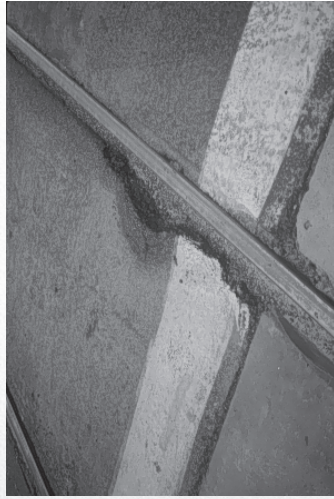
Figure 16-12. POTENTIAL PROBLEM: Broken surfaces should be avoided at railroad crossings. A surface material that will not buckle, expand, or contract significantly should be used near railroad tracks.
