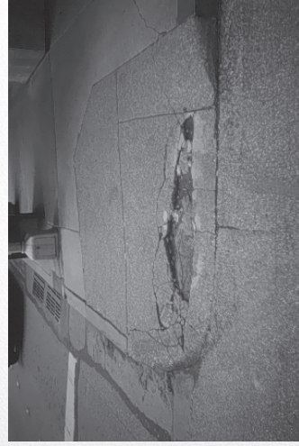
Figure 10-2. Sidewalk cracks and broken concrete are common sidewalk maintenance problems that inhibit pedestrian access to sidewalks.
