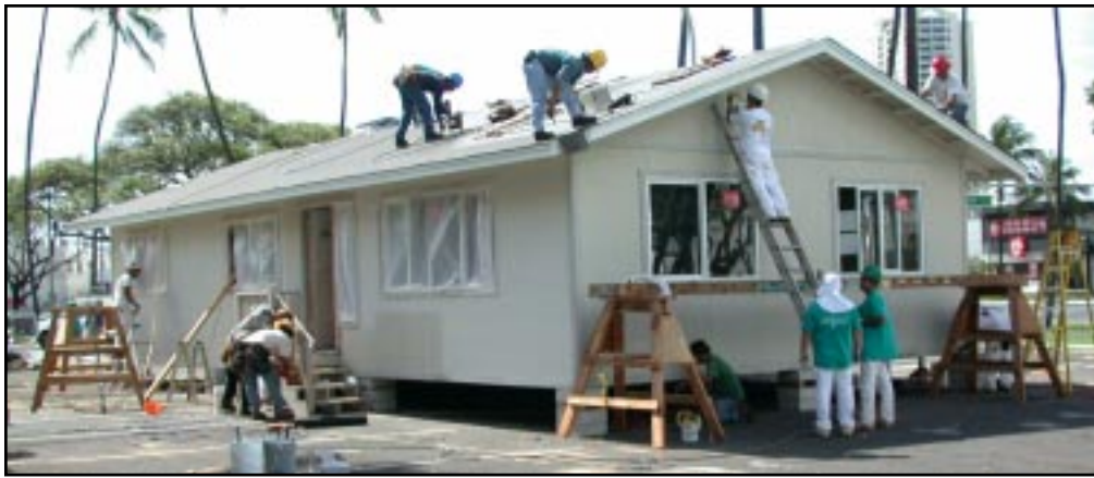
Figure 4. The steel-framed Speed House not only was erected in a single day, but featured insulated radiant barriers, a solar water heater, a roof ridge vent, vented eaves and other efficiency features.
