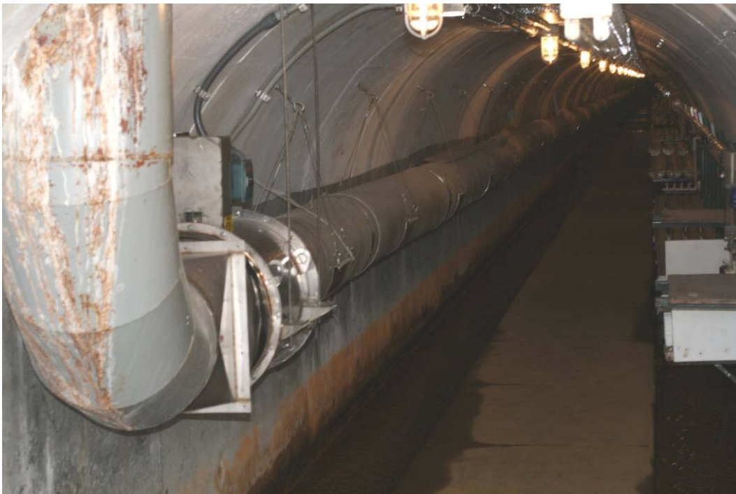
Figure 19. Photograph taken on March 25, 2008 looking upstream from the Portal area in the LMDT showing the ventilation fan, motor controls, and vent pipe at left, and the electric lights at the upper right.
