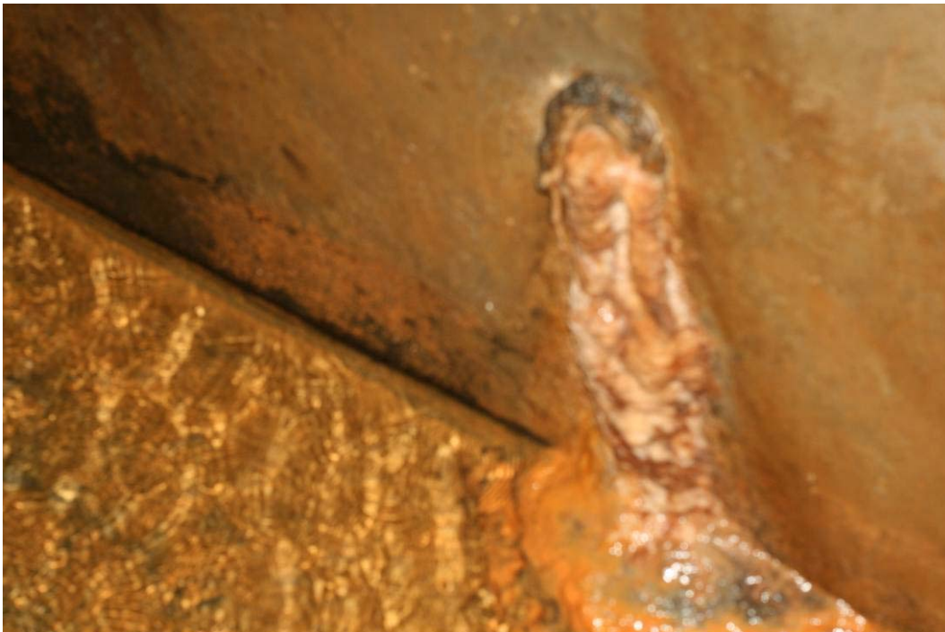
Figure 22. Photograph of a weep hole in the reinforced concrete lining which is almost completely blocked by calcium carbonate precipitates.
