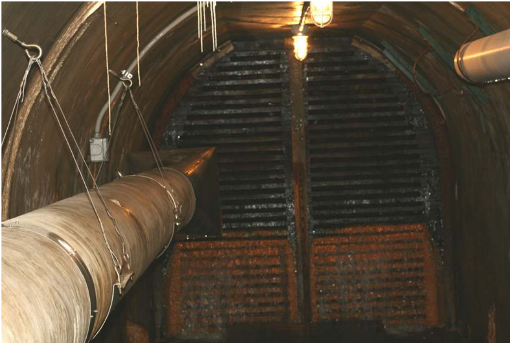
Figure 23. Photograph taken on March 25, 2008 of the cobble and gravel-filled timber-lattice bulkhead at Station 4+61 of the LMDT. At left is the intake end of the ventilation pipeline.
