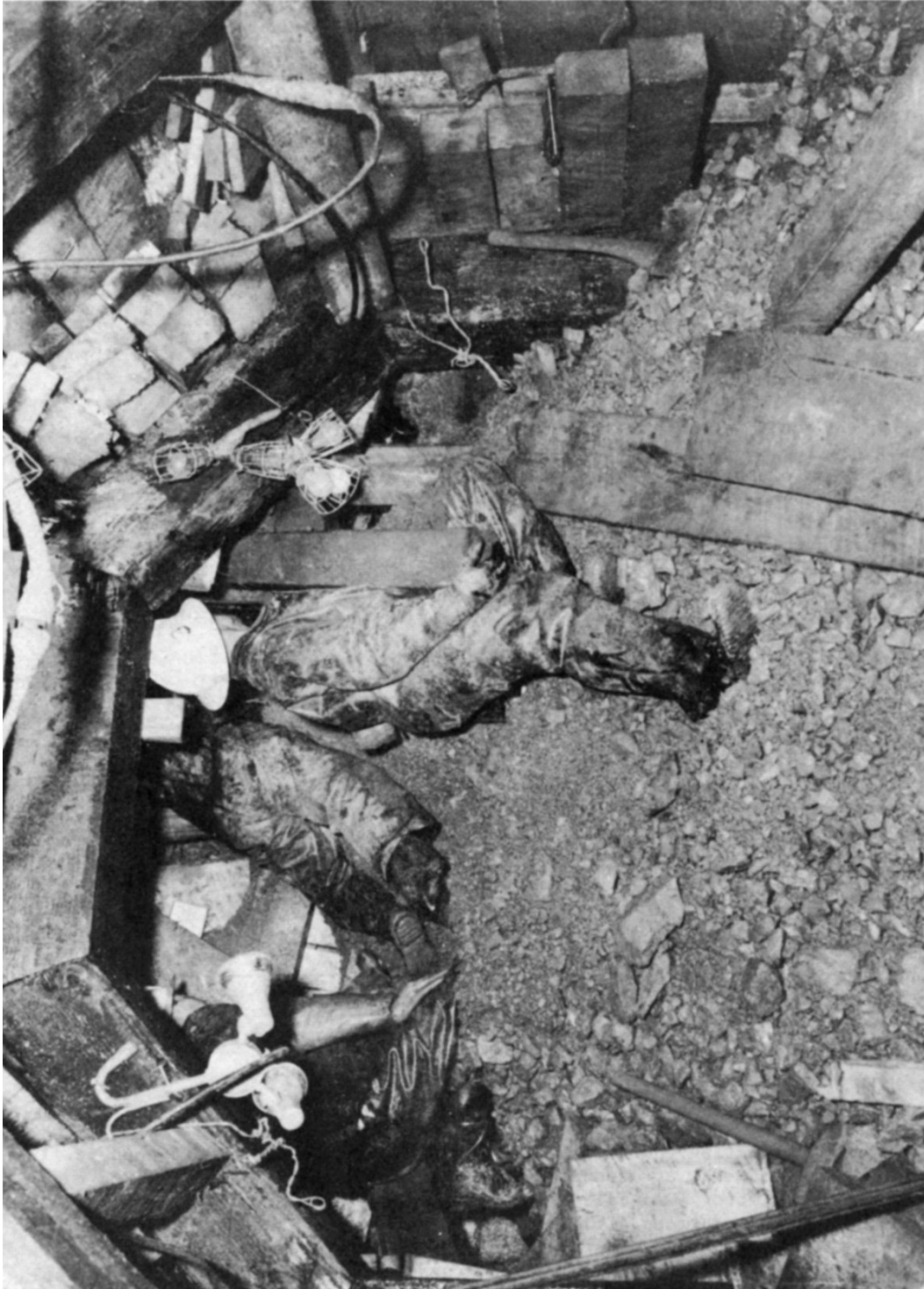
Figure 13. Workers digging out a boulder embedded in running ground in sheared quartzite, taken from (Salsbury, 1956). The boulder prevented spiles from being driven.
