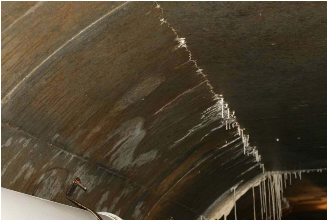
Figure 20. Photograph taken on March 25, 2008 looking downstream from about midway inside the reinforced concrete lined segment of the LMDT. Note the calcium carbonate stalagmites forming from the slow seepage along a thin roof crack and at a joint in the concrete lining.
