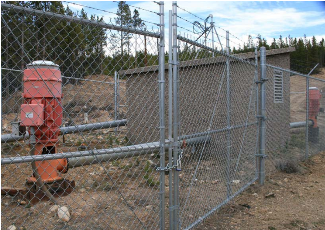
Figure 29. View of Pumphouse and Extraction Wells in the vicinity of Station 10+25. May 28, 2008.
