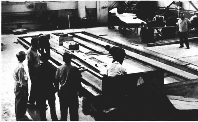
The concrete pit and steel rails (here covered with wood for protection).
