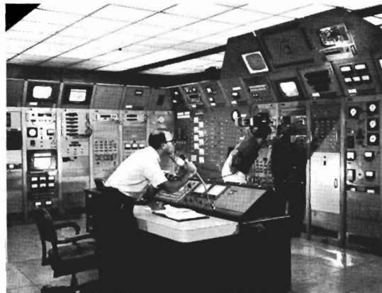
MAIN CONTROL ROOM
