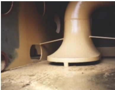
Figure 1: Ballast pump intakes are typically located a few inches off the tank floor resulting in the accumulation of residual water and sediment after the tanks have been emptied. Photo credit: Captain Phil Jenkins.
