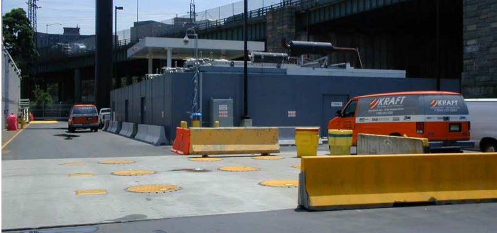
Figure 4. CNG Compression Station at West Farms Depot
