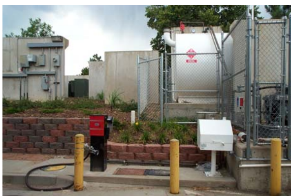
Figure 2. B20 Fueling Station
