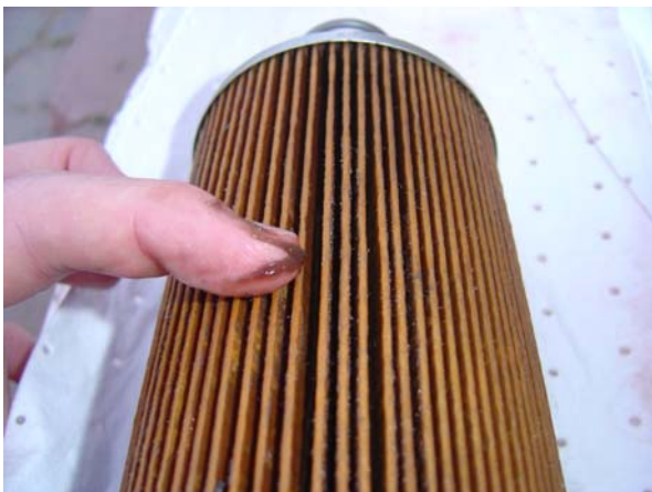
Figure 9. Bus 2210 Plugged Filter Examination
