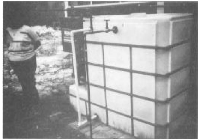
Second View of Pump & Storage System
