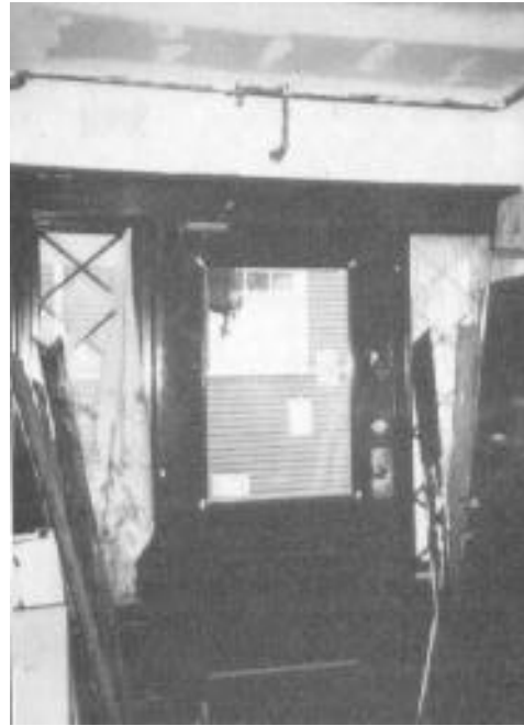
View of front door depicting branch to front porch where a freeze-proof dry pendent was employed.
