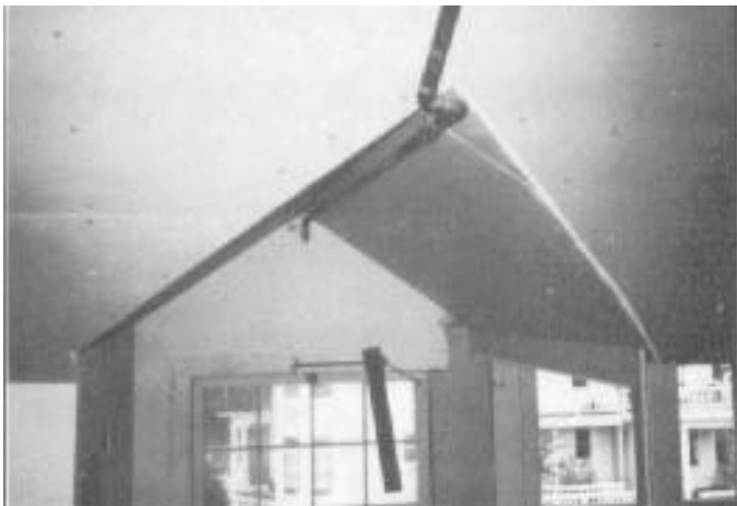
Sprinkler in Dormer in Top Floor Apartment. This unit was deemed a habitable space-by SFD because of the installation of fire sprinklers.
