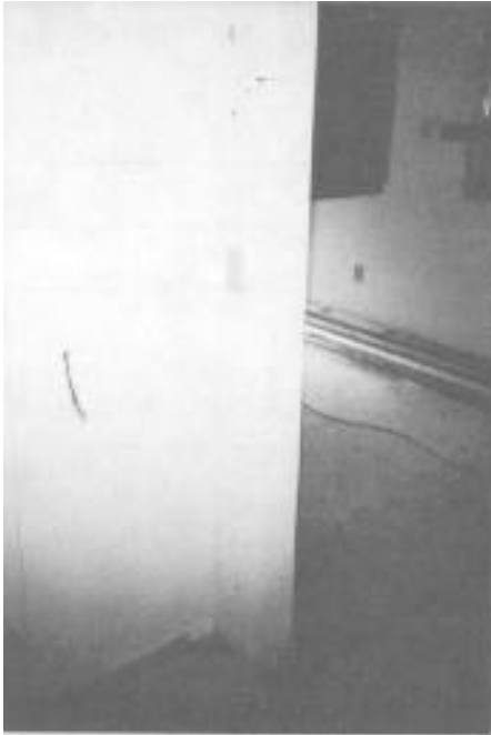
Rehabilitation of North Marks Street House included measures taken to enhance accessibility to wheelchair occupant. Shown here is a wall switch lowered to 42 inches.
