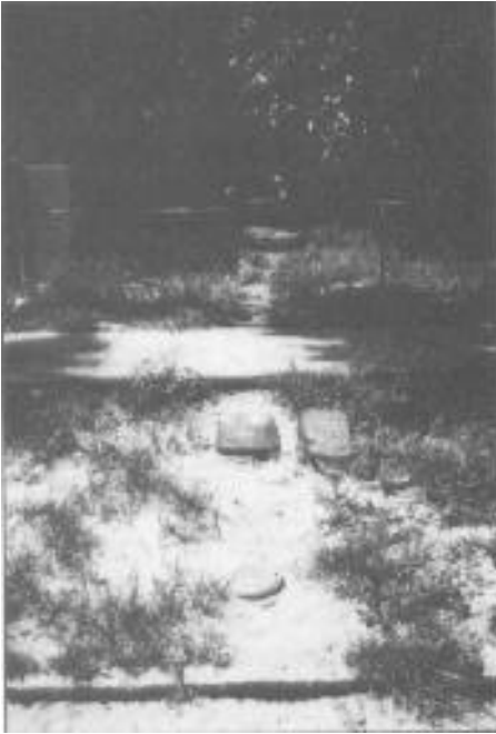
Some Water Departments Require New Metered Water Supplies to Sprinkler Systems. New Meter Box is Shown Here Adjacent to Existing Meter.
