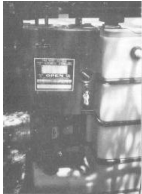
Control panel for pump & storage system.
