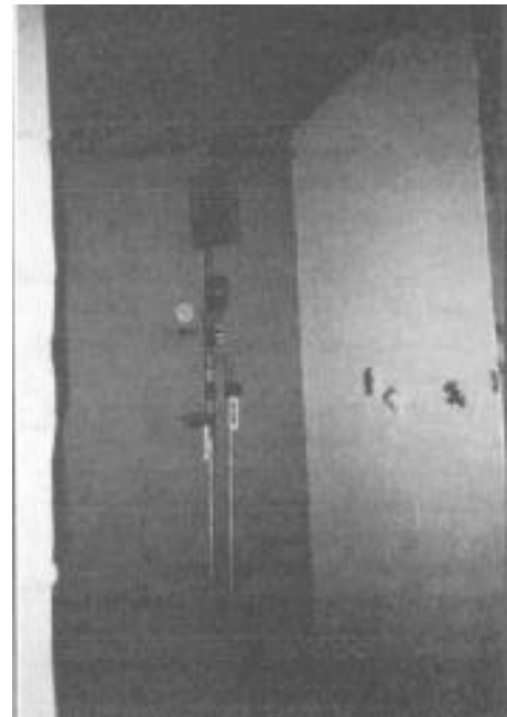
Water service to Sprinkler System, with valve tags and user's guide
