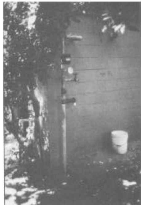
New Water Service for Sprinkler System at 11th Street Home. Supply valve was locked with lock and chain to prevent valve closure.
