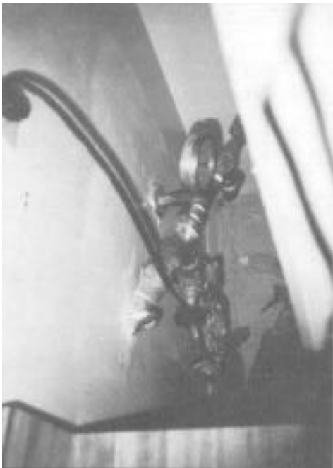
Control Valves at Miller St. house were located behind the refrigerator to discourage tampering.
