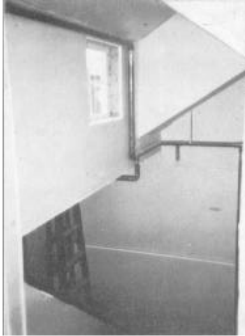
Pendent Sidewall Sprinkler Head Located in Staircase to Upper Apartments
