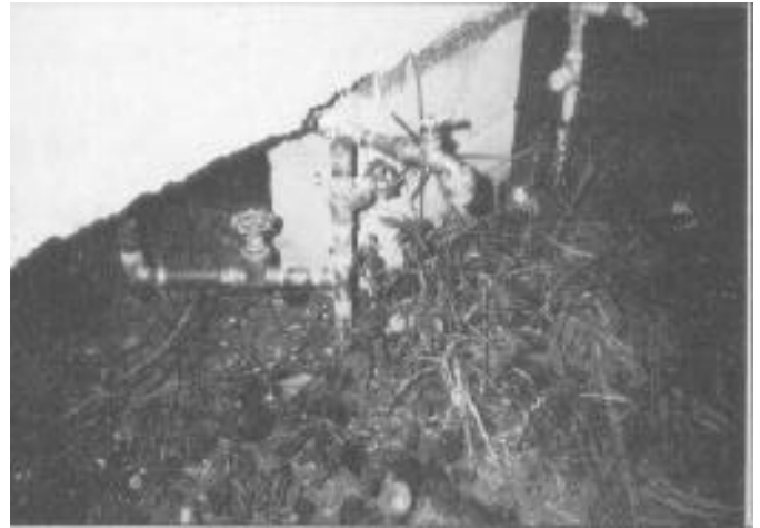
Exterior View of Sprinkler Water Connections at Miller St. Home.
