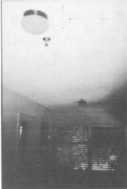
Typical Finished Ceiling with Conventional Pendant-Type Sprinkler Head
