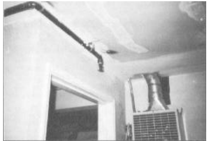
Pendent Sidewall Sprinkler Head in Furnace Area. Pendent sidewall heads were used throughout most of the Victoria Apartments.
