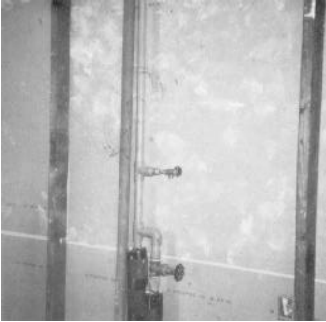
Tied together water supply with shutoff and test valves.
