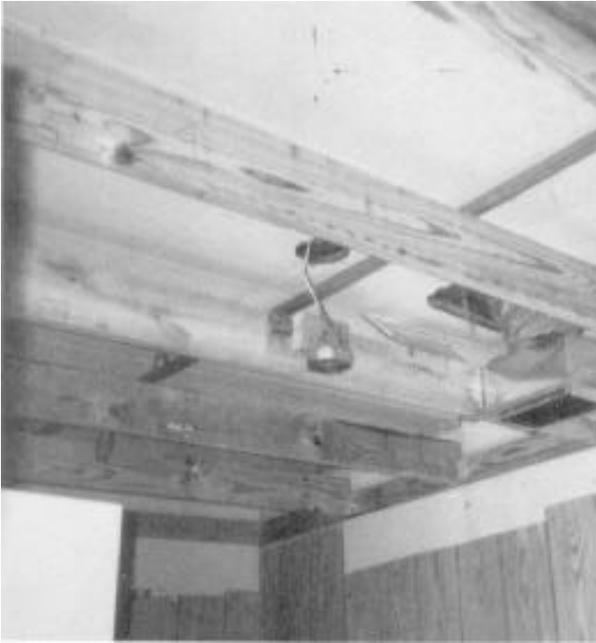
Lateral pipe with sprinkler connections in ceiling.
