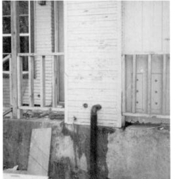
Water connection from city water main, and sprinkler drain pipe (2601 Sol Wilson).
