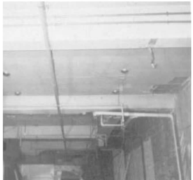
Sprinkler system laterals in commercial area.
