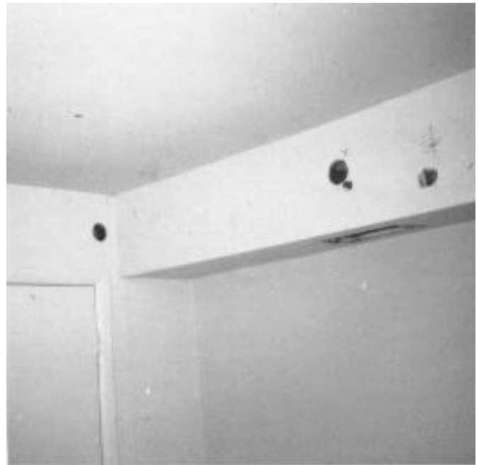
Holes cut for sprinkler piping through heating duct.
