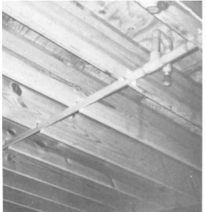
Sprinkler system through joists.
