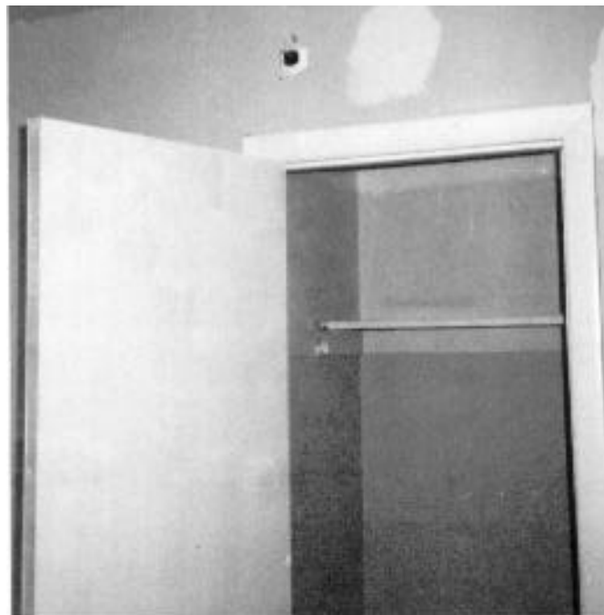
sidewall head not in soffit, above closet.
