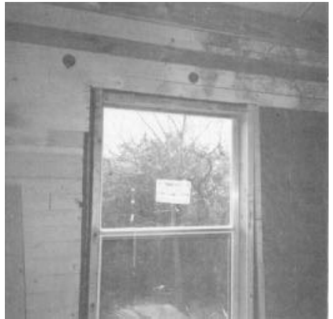
Interior of 3501 Pennsylvania Avenue during rehabilitation with new window and insulation installed in walls.
