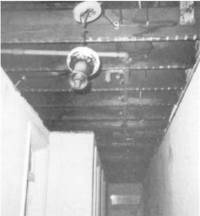
rafters system lateral piping and head fitting cut through ceiling
