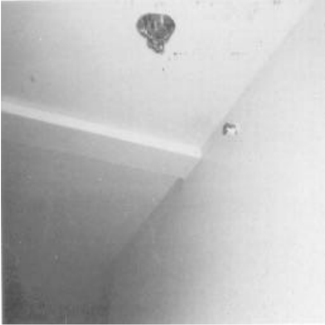
Sprinkler System Plumbing
