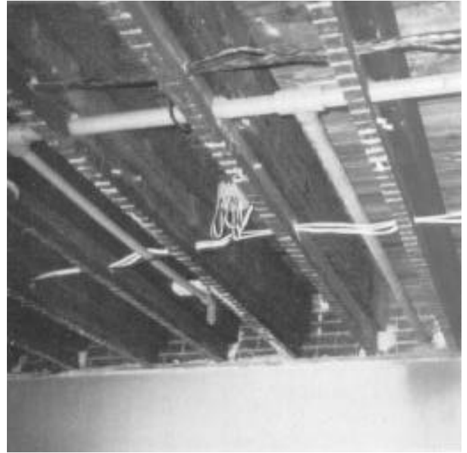
Sprinkler system "t" connections adjacent to electric conductors in ceiling rafters.
