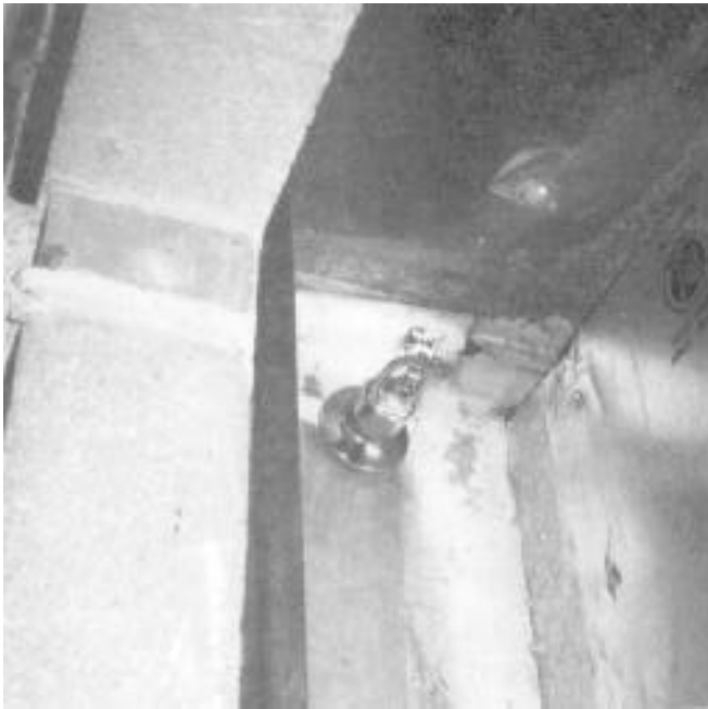
Typical sidewall dry sprinkler head in furnace closet.
