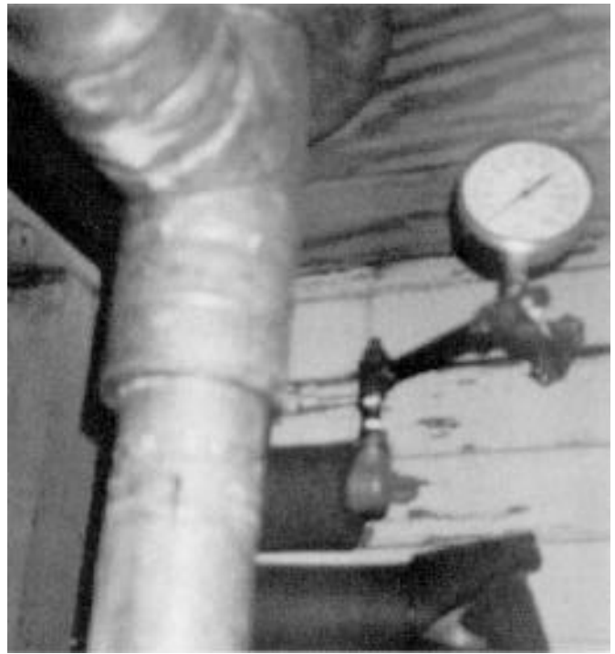
View of control manifold with back-flow preventer, drain and test valves, and pressure gauge, in heater closet at 2601 Sol Wilson.
