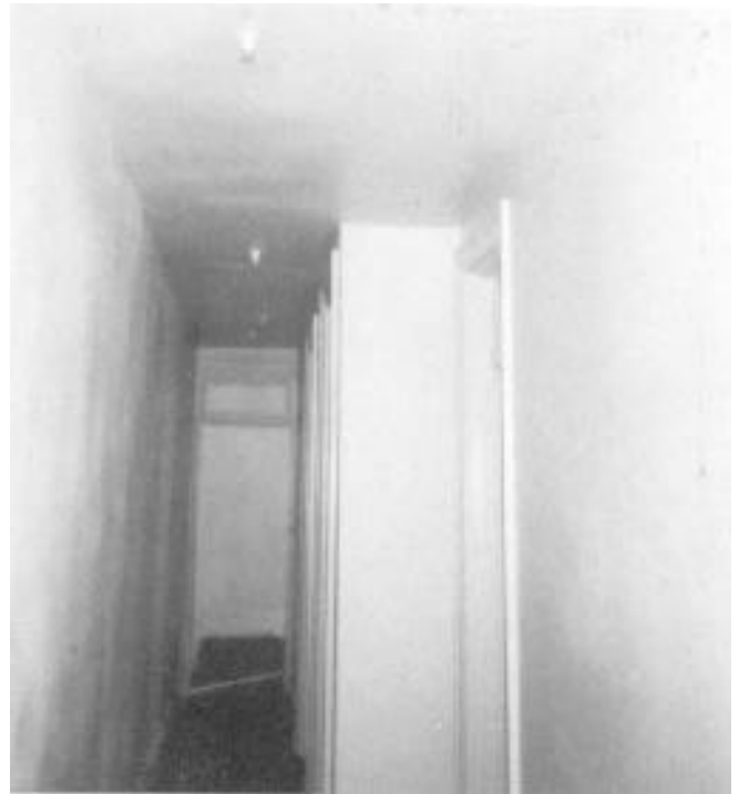
Pendant type sprinkler heads (capped) in finished interior hallway,
