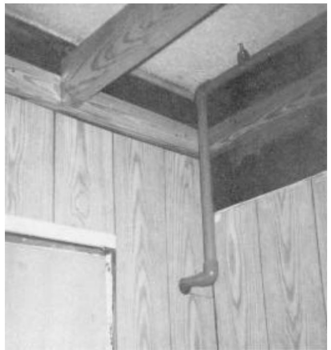
Sprinkler runs before relocating behind wall (2601 Sol Wilson).
