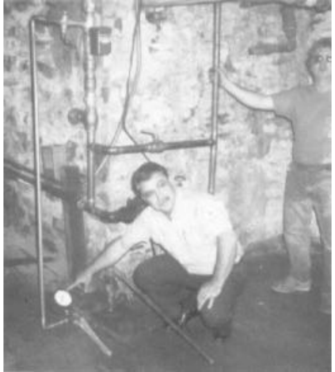
Chief Larry Stamer, Harrisburg Bureau of Fire Safety certifying pressure for system static pressure test.
