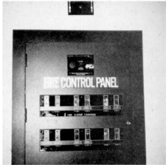
Fire Control Panel.
