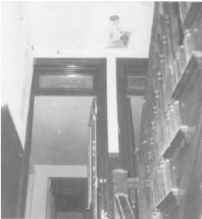
Sidewall sprinkler head in common hall, ceiling sprinkler head in entrance foyer of apartment.
