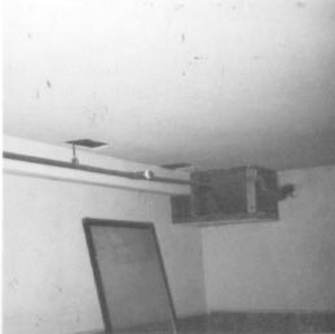
CPVC piping wrapped around hot air duct work.
