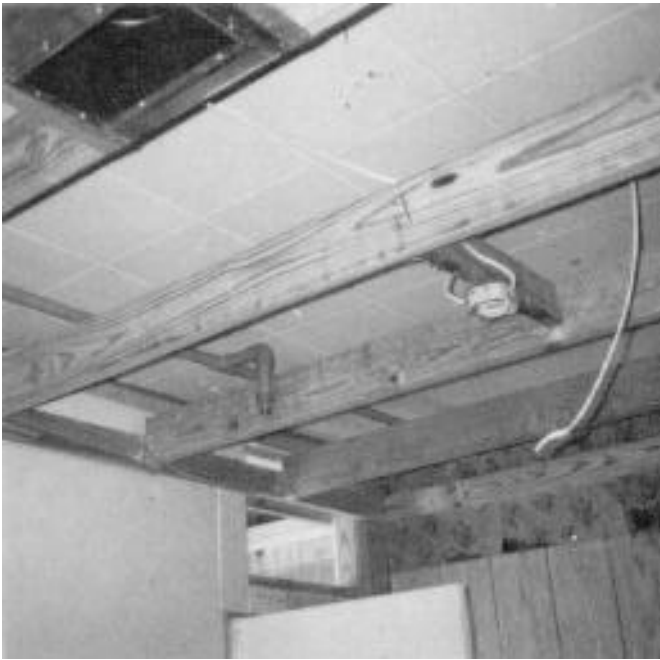
Sprinkler connections and other utility connections (2601 Sol Wilson).
