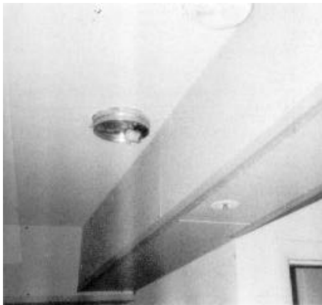
Ceiling pendant head between rooms, with smoke detector and ceiling light fixture.
