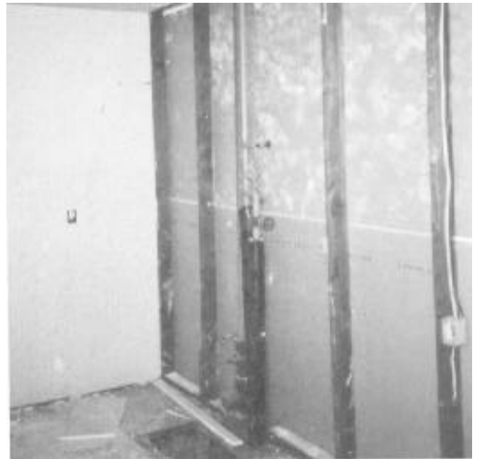
Domestic water supplies tied together into one supply for sprinklers (3501 Pennsylvania Avenue).
