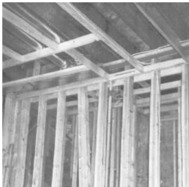
Sprinkler system riser, laterals, and heads "Blazemaster" CPVC Piping-
