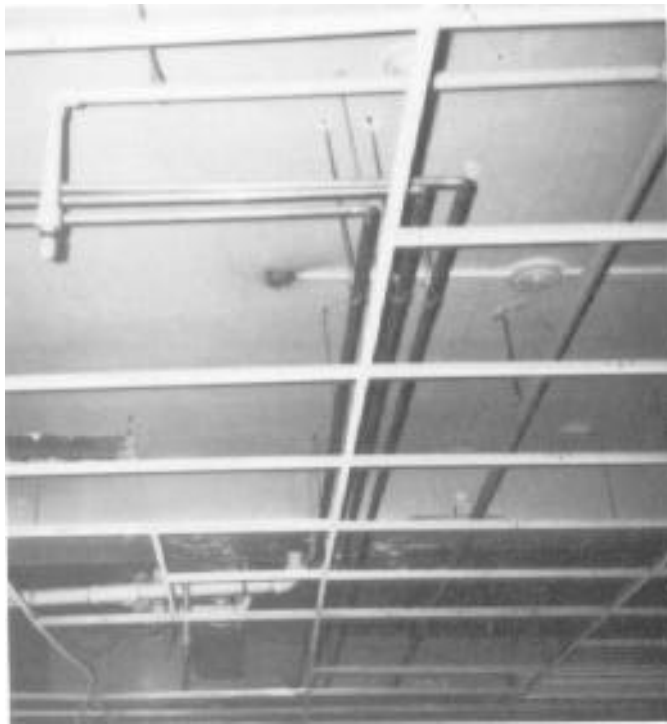
Sprinkler system laterals and elbows adjacent to other building utility systems.
