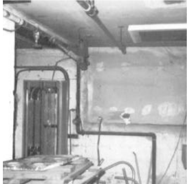
Utility and laundry area with commercial sprinkler system.
