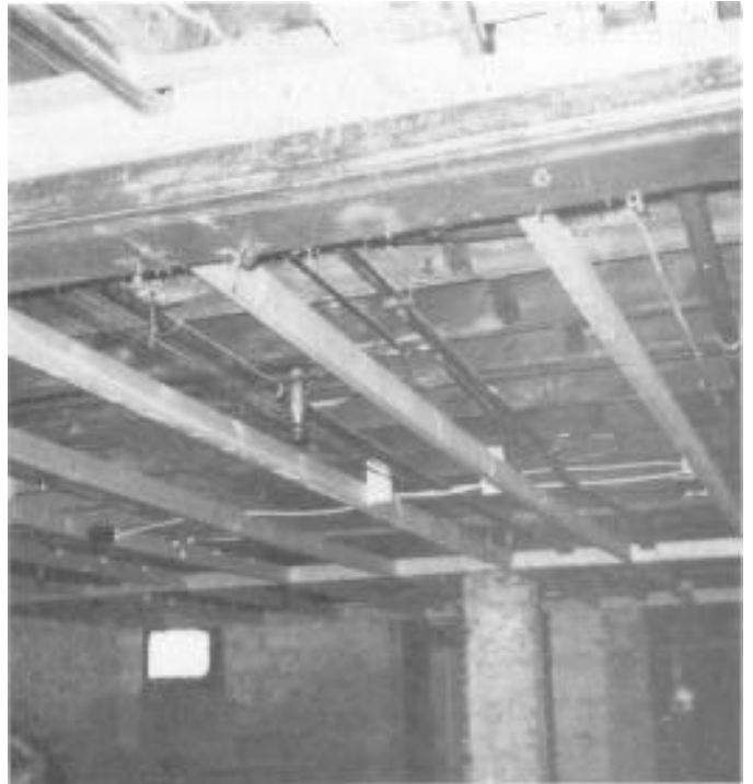
Sprinkler heads in basement ceiling, and Don Bollinger of St. Louis Community Development Agency.
