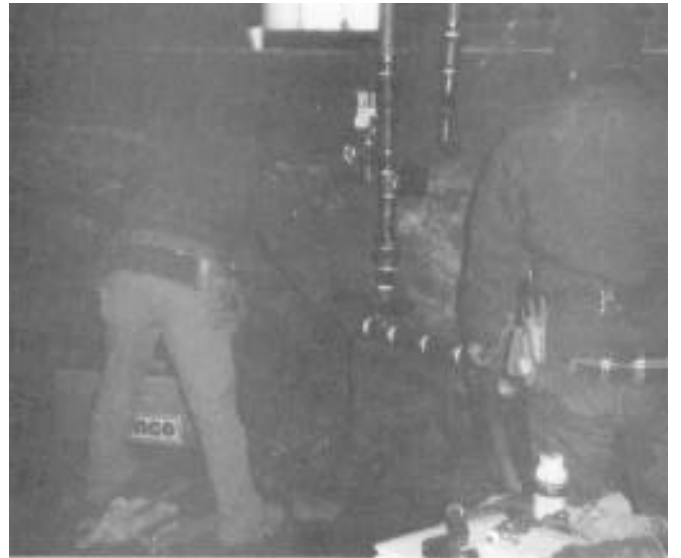
Double check valves, flow alarm switch, pressure gauge, and drain valve located at water service connection.
