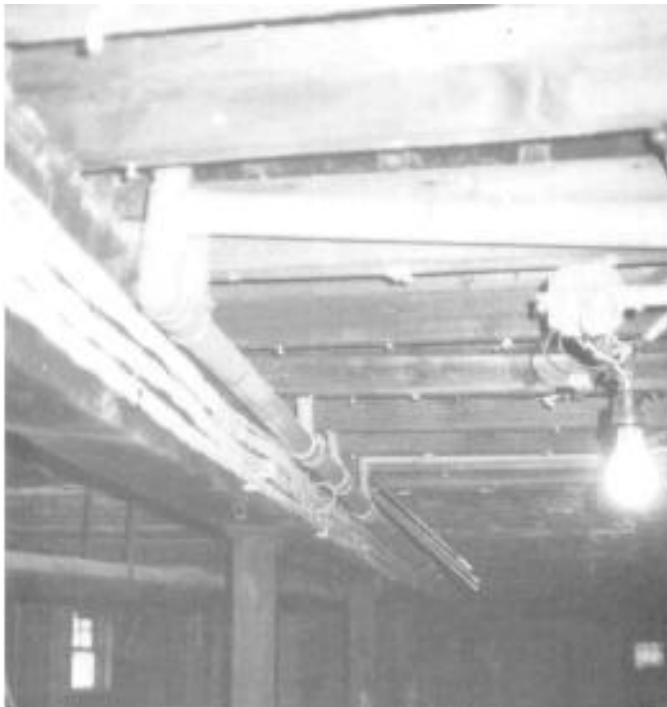
Adjacent horizontal laterals, sprinkler and electric systems.
