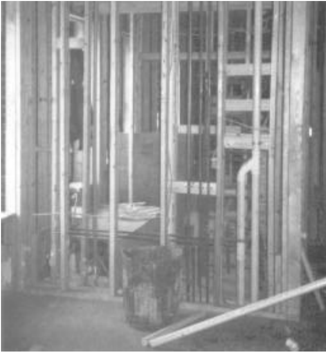
Adjacent risers, sprinkler system, domestic water, waste and vent.
