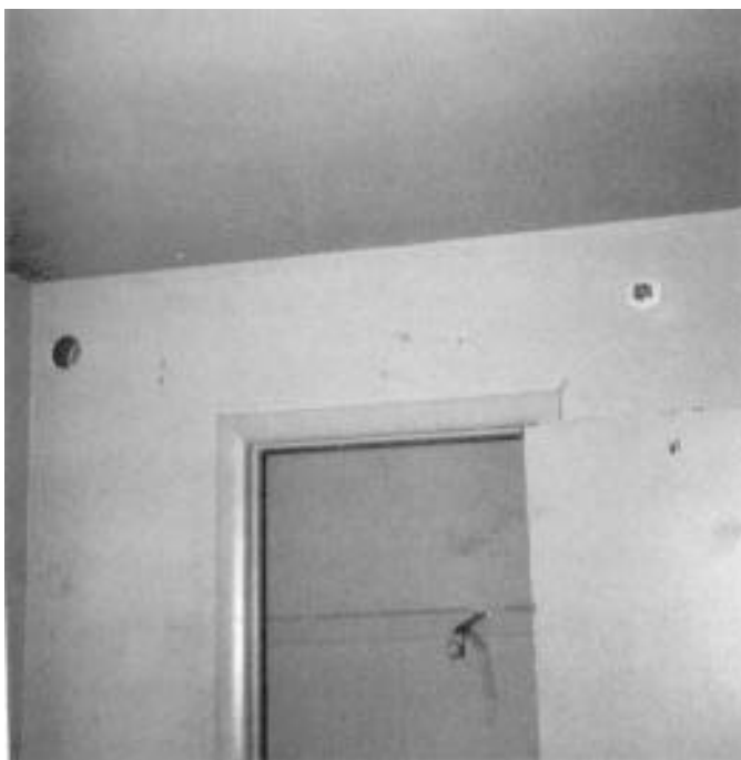
sprinkler head, above closet, during rehabilitation.
