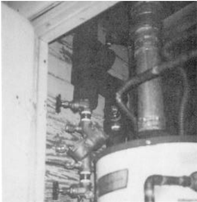
View of control manifold with back-flow preventer, drain and test valves, and pressure gauge, in heater closet at 2601 Sol Wilson.
