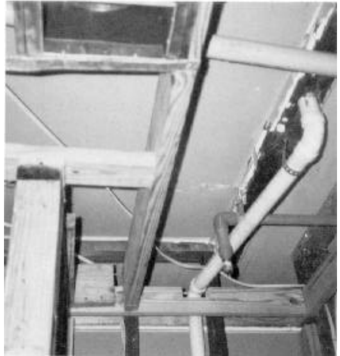
Adjacent water systems, sprinkler, and domestic sanitary vent stack (3501 Pennsylvania Avenue).
