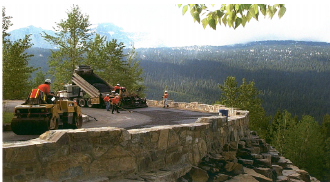
Before and after road repairs at Glacier National Park in Montana. Maintenance can enhance safety and the beauty of national parks.
