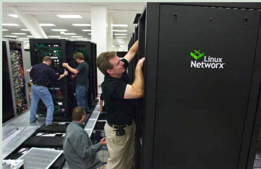
Workers install the Jacquard cluster cabinets in NERSC's machine room. The system provides 640 processors for scientific computing.
