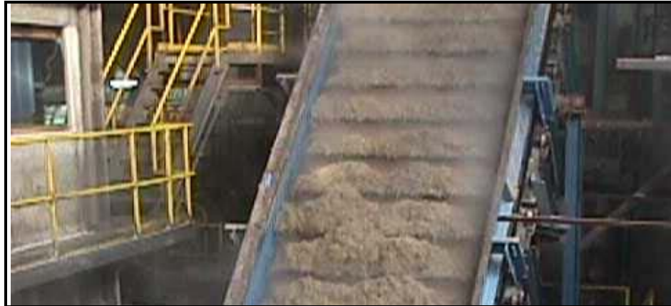
Figure 14 Bagasse Conveyed to Storage
