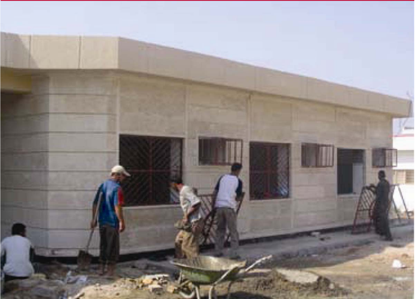
The new primary health center (PHC) building, which is currently being constructed by UNICEF using USAID funds, provides health services for a population of 12,283 (of which 2,900 are children under five years of age).
