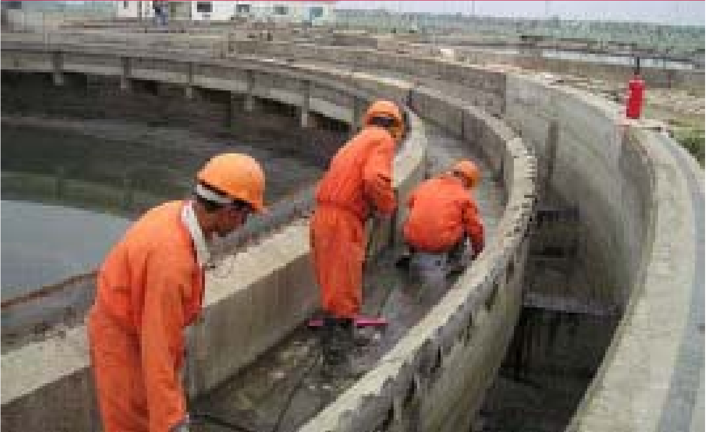
Iraqi workers repair joints at the Rustimiyah North wastewater treatment plant in Baghdad.
