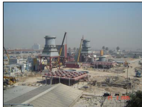
Baghdad South power plant
