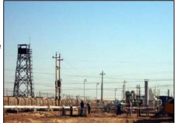
Two new power generators at the Kirkuk substation will add 325 MW of power .
