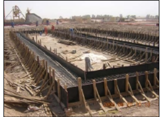
Laying a foundation at the new water treatment facilities in Sadr City, Baghdad
