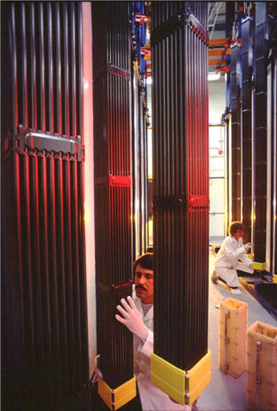
Figure 13: Typical Fuel Assembly Storage (UO2 - MOX storage is similar)
