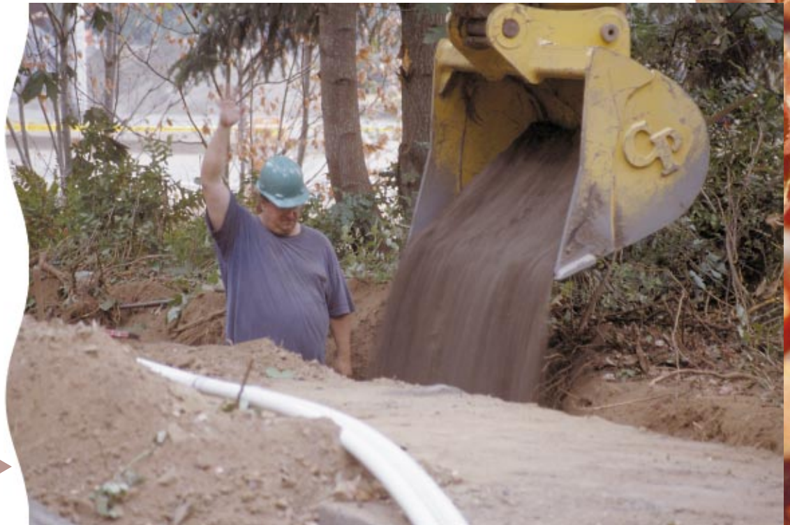
New sewer lines connect the existing storage tanks to the new drain field.
