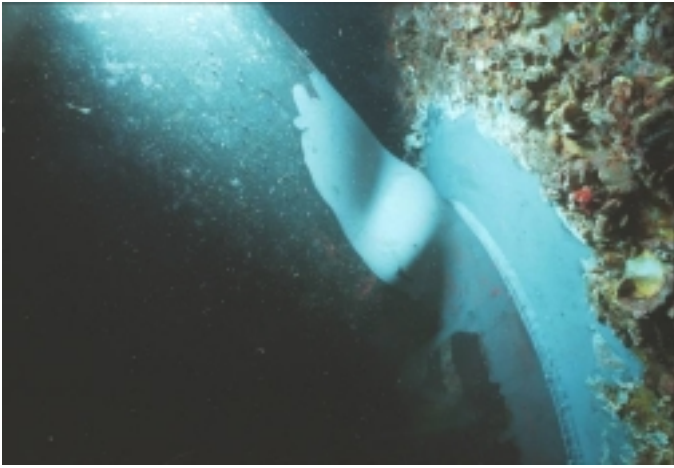
Figure 5 – Local Buckle of a Brace near a Joint
