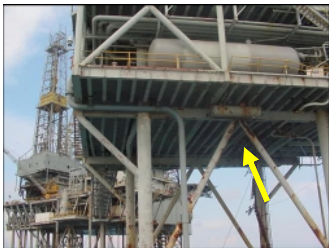
Figure 10 – Bent Beams Under Deck
