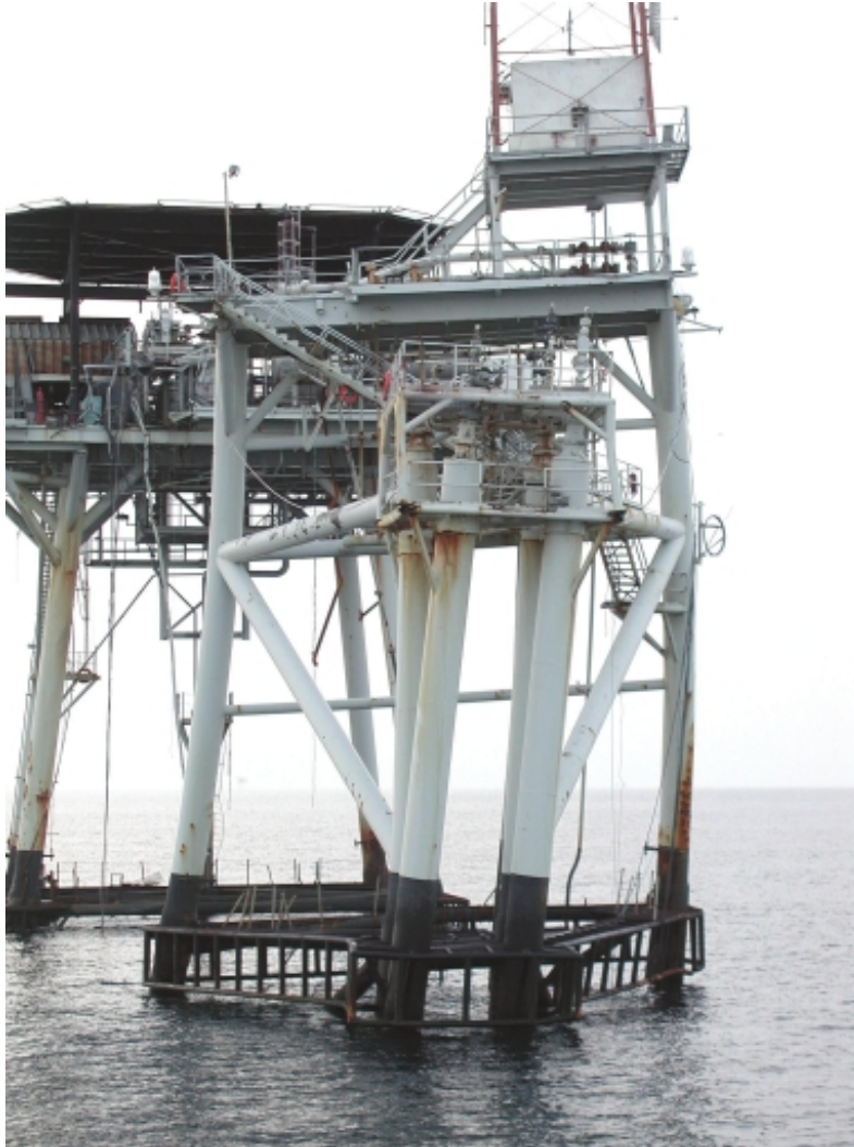
Note the gross permanent deflection of the structure in this post storm photograph of EI-231-CA
