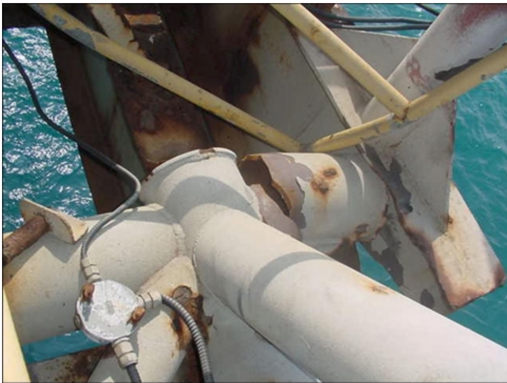
EI-295-A-PRD bridge damage is shown here after the storm. Note the cracked brace in the center of the photo. The bridge deflected several inches during the storm.
