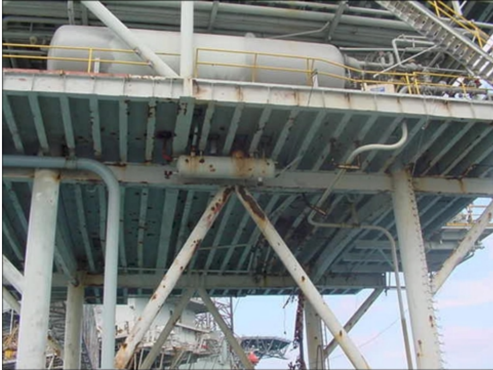
EI-295-A-PRD deck damage is shown here after the storm. Note the deflected beams on the underside of the deck.
