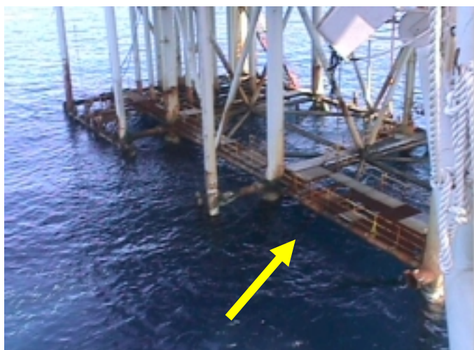
Figure 9 – Missing Boat Landing
