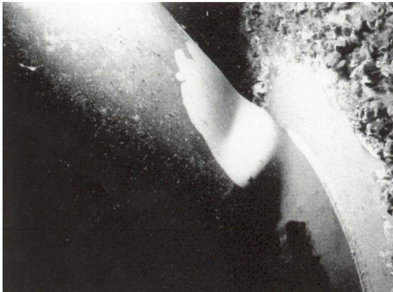
EI-276-B-Aux damage identified during subsea survey after the storm shows buckling to vertical diagonal brace.
