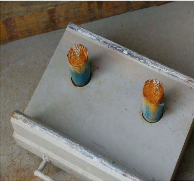
Figure 8 – Sheared bolts in Ram Powell rig hurricane clamps
