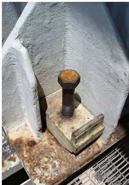
Figure 2 – Loosened Bolt for Tie-Down
