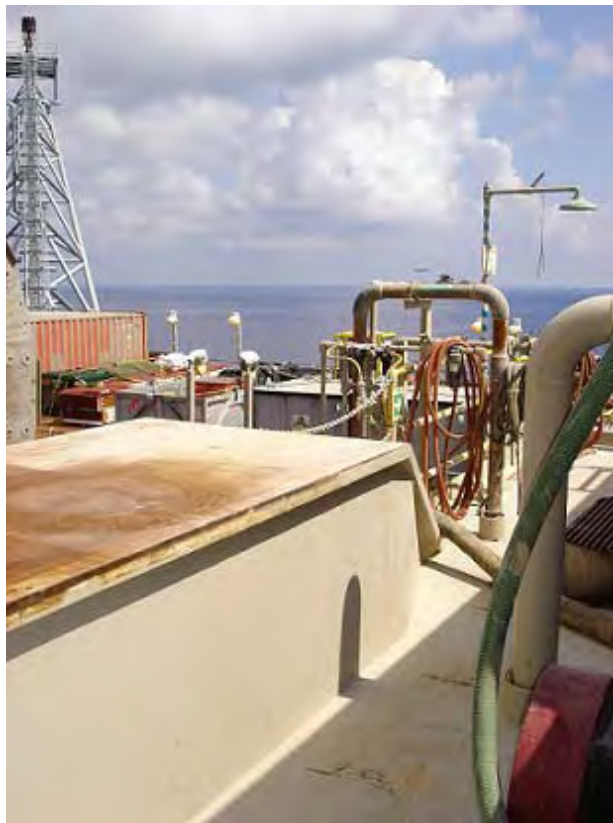
Figure 6 - Skid for Holstein Substructure
