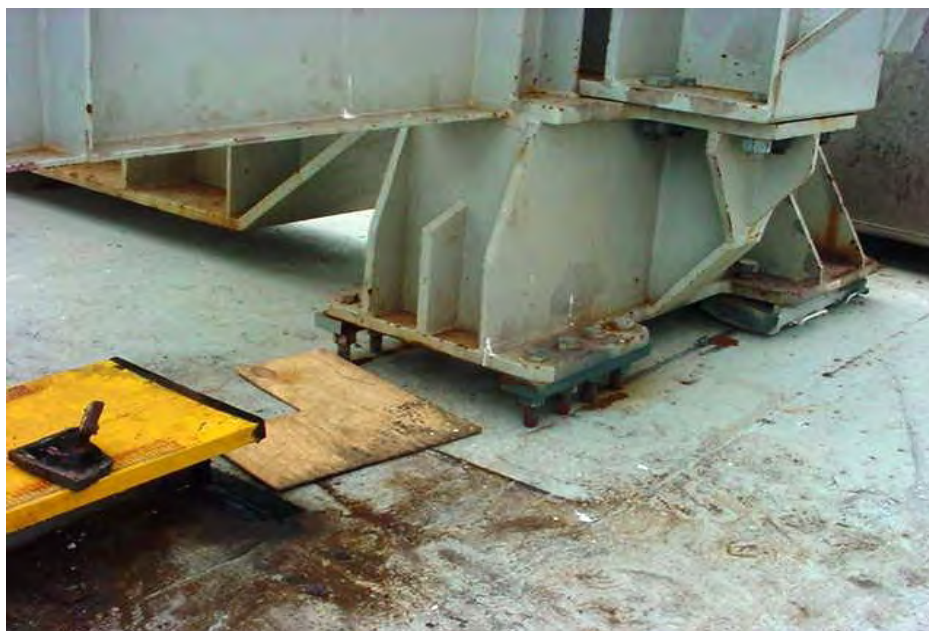
Figure 16 - Horn Mountain Rig Skid Beam Damage From Hurricane Ivan
