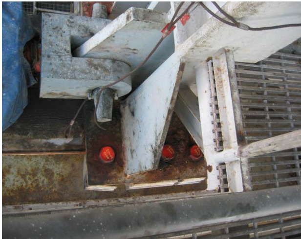
Drill Floor to Skid Beam
