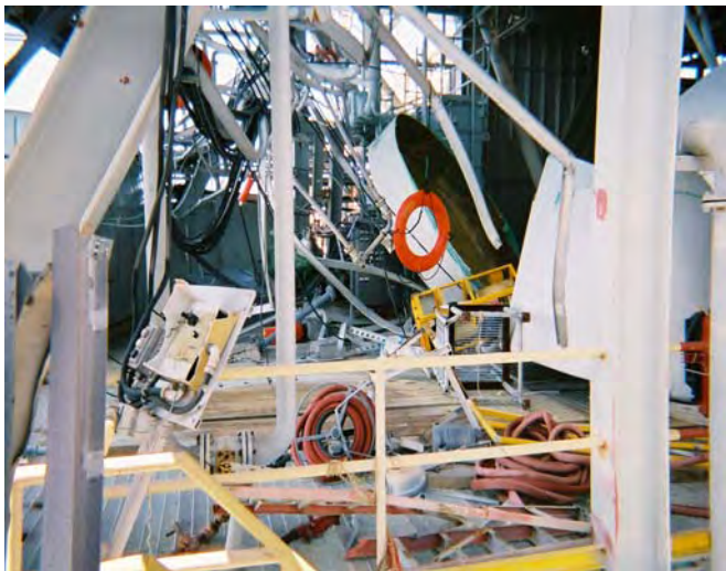
Figure 10 – Main Pass 252 damage
