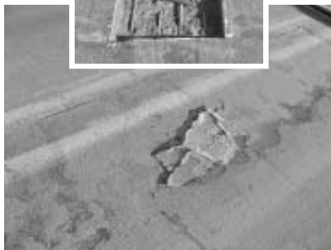
Condition of bridge deck on Biggs Bridge.
