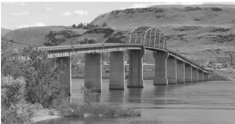
Washington DOT repairs of the US97 Biggs Rapids - Sam Hill Bridge over the Columbia River requires closing the bridge, sending motorists and truckers on a substantial detour around the work.
