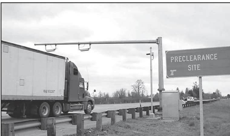
Transponder readers mounted on a mast arm extending over the roadway look for signals from transponders on truck windshields. Since transponders can't be turned on or off, the readers will recognize every transponder's unique identifying signal. If a particular transponder is not enrolled in the system and linked to any company's records, the driver will see a red light on the transponder indicating he or she must stop at the weigh station.
