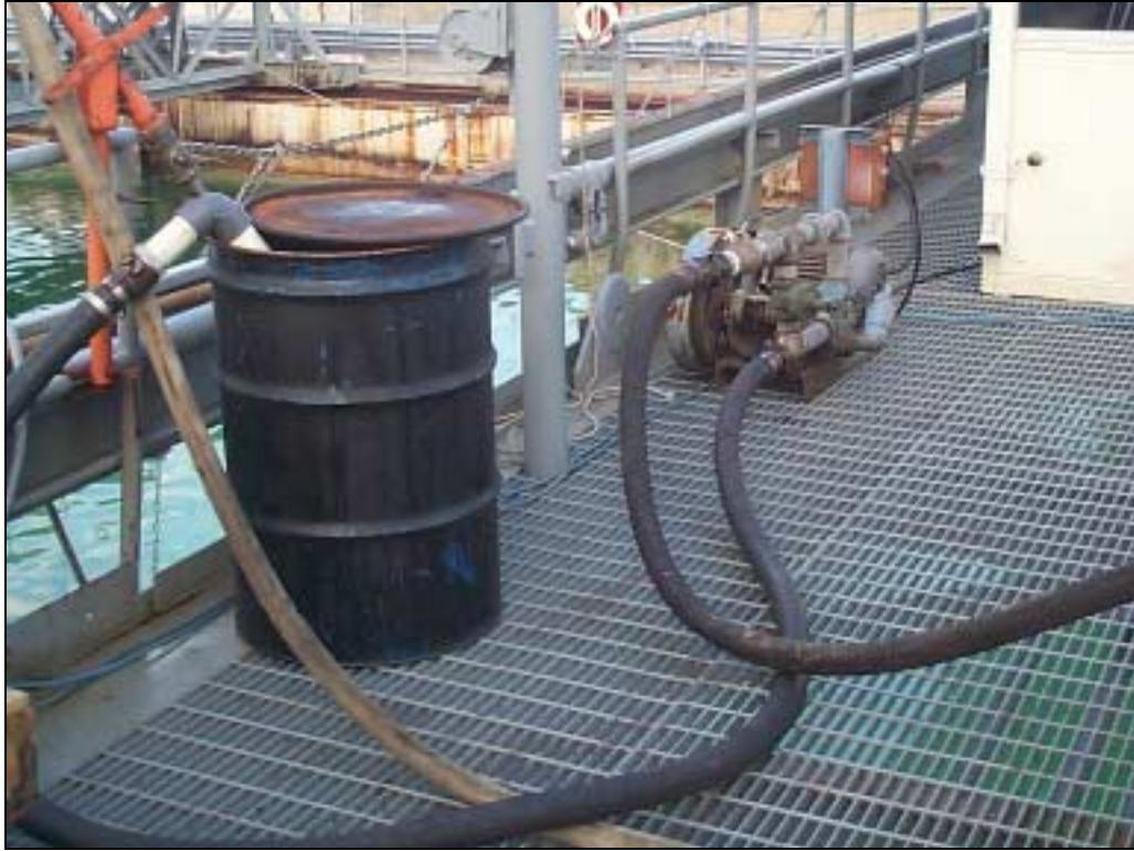
Figure 6. Oil Delivery Pump and Supply Drum
