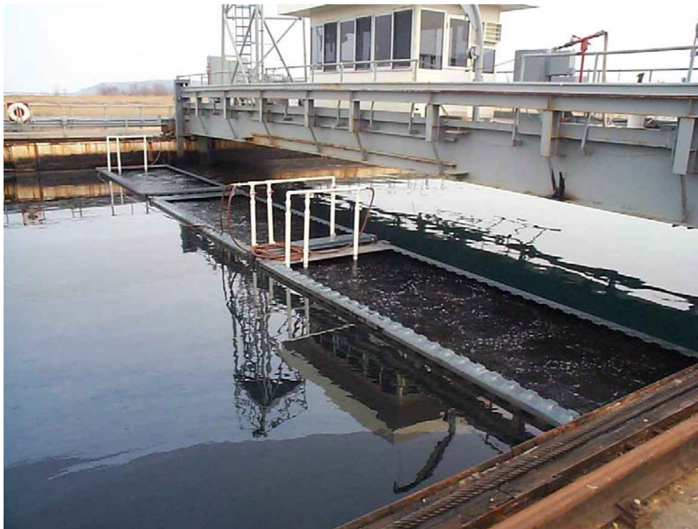
Figure 20: System in operation.
