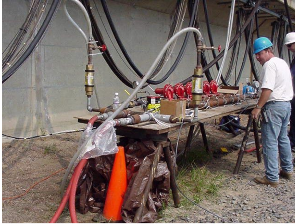
Figure 4. Propane regulators and compressed air control valves.
