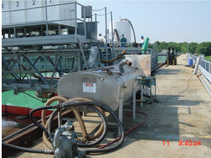
Figure 5 Steel Temporary Holding Tank for Decanted Water
