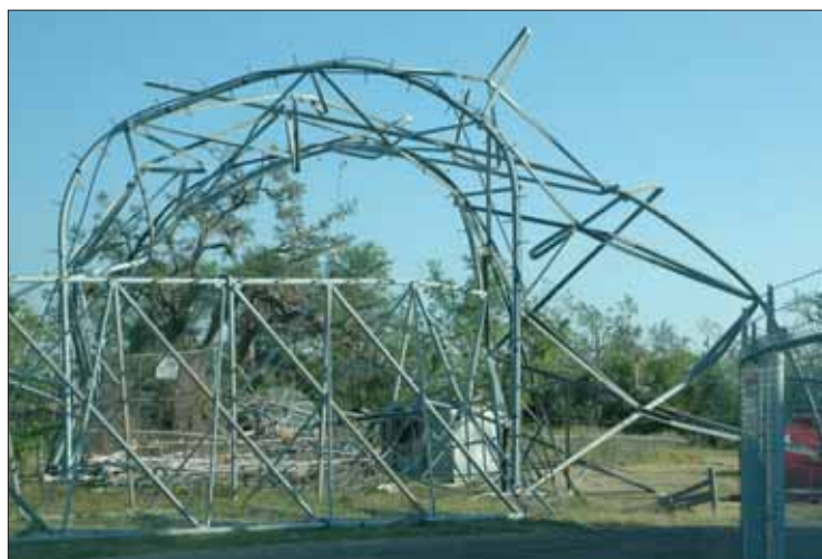
A downed communications tower, Plaquemines Parish, LA.
