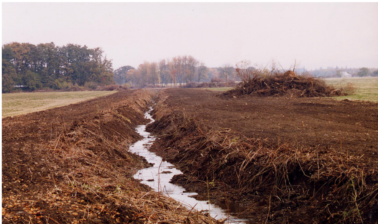
Ditching of slope/flats wetlands removes capacity to store water and can thus aggravate downslope flooding and water quality problems. (photo courtesy of Tom Moser)
