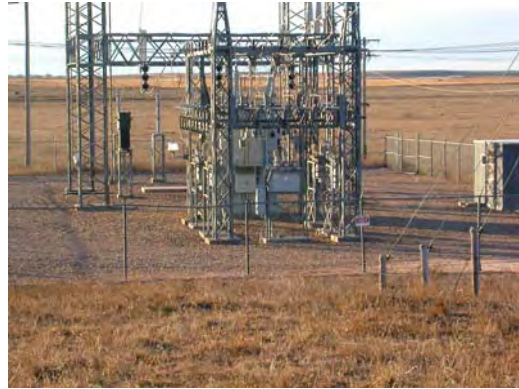
Typical HEA Distribution Substation
