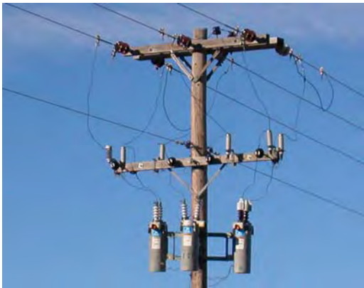
Three Single-Phase Reclosers
