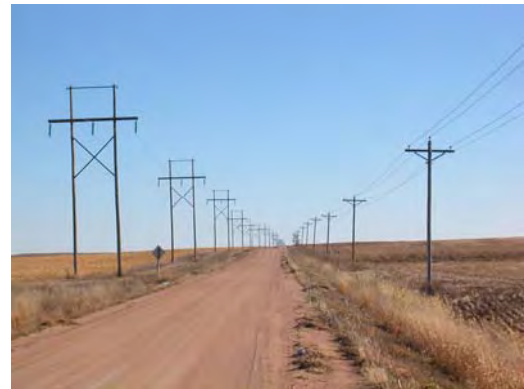
115 kV Transmission Line and 3-Phase 12.47 kV Distribution Line
