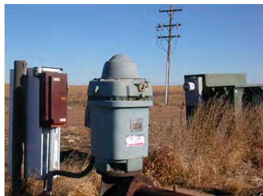
100 HP Irrigation Pump with Pad-Mounted Transformer and Meter
