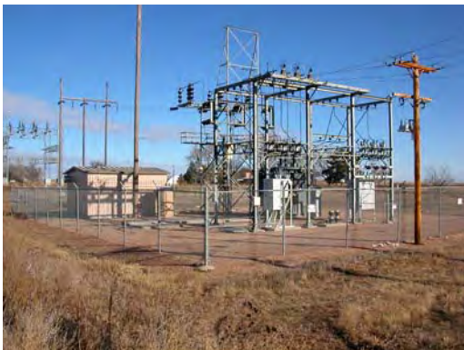
Julesburg Distribution Substation
