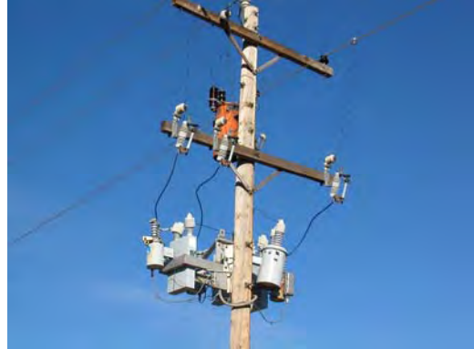
Three-Phase Capacitor Bank
