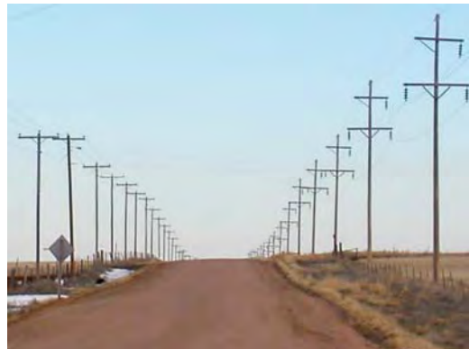
12.47 kV 3-Phase Distribution Line And 69 kV Transmission Line
