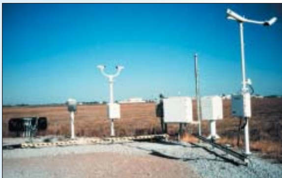
Automated Surface Observing System (ASOS).
