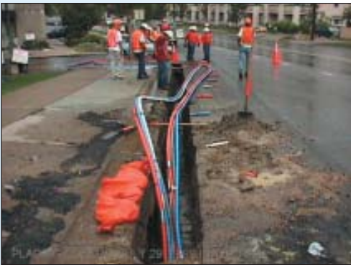
Placing conduit for the Boulder (Colorado) Research and Administrative Network, a fiber optic network that supports networking research and technology. The project was supported by NOAA's HPCC program.
