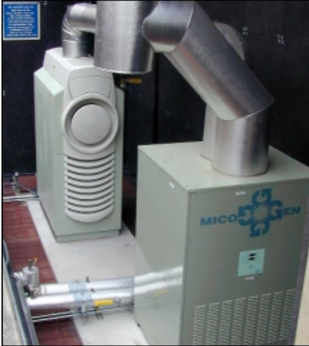
The microturbine recently installed at the CU, Boulder Recreational Center.
