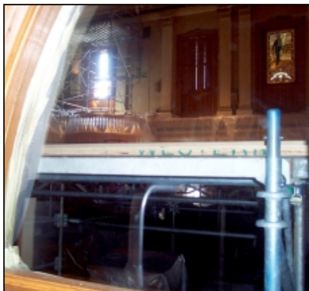
The false floor that was erected in each of the legislative chambers. The desks and chairs are under the floor you see in the middle of the picture, while the construction crews work above installing smoke detectors and sprinkler systems.
