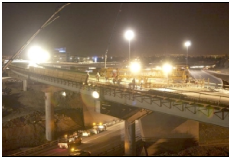
Much of the T-REX work takes place at night in order to limit the impact on traffic flow. Pictured above is the installation of the flyover from southbound I-25 to northbound I-225.
