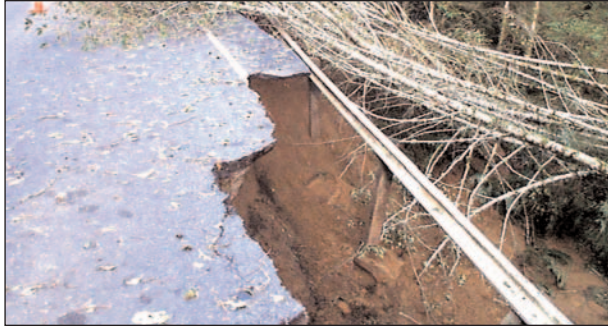
Our department is part of an interagency group to provide early warning of landslide dangers in Western Oregon. (Photo: Oregon Department of Transportation)
