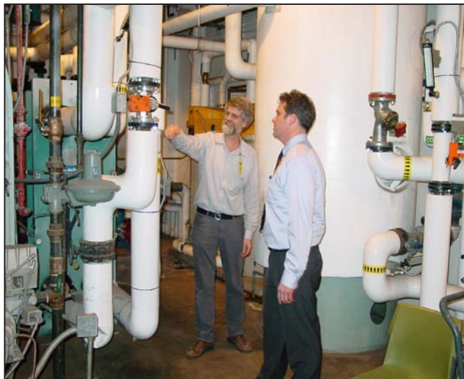
Project engineer Brian Brown P.E. (left) shows Energy Analyst Brian Herbstrith with the Oregon Department of Energy the modulated control valves for the Henley High geothermal HVAC heating system.
