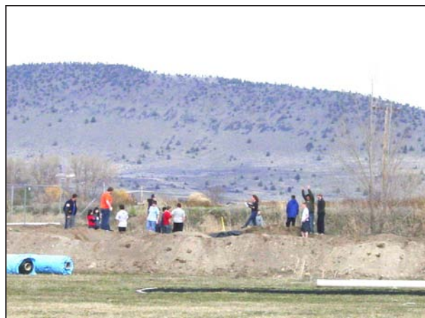
Students at Henley High are working at constructing a pond with the geothermal water used to heat the school. The pond, located near the football field, will be used as an outdoor lab for biology students.
