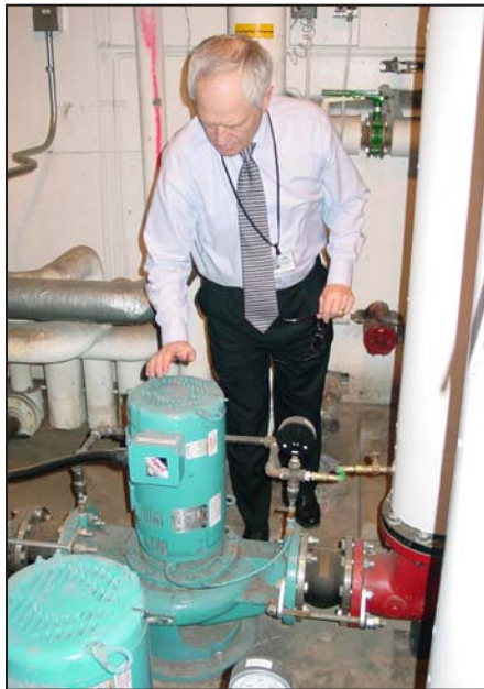
Klamath County School District Business Manager Ken Hadlock shows off a new circulation pump at Henley High.
