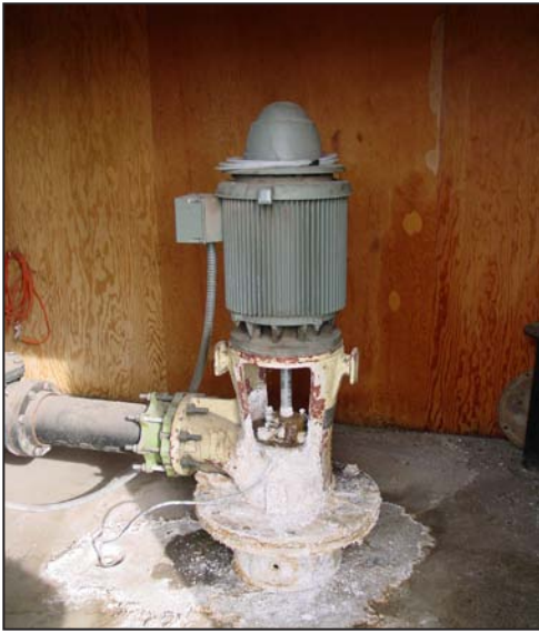
The well that pumps the geothermal water to Henley High is in a small mechanical shed next to the football field.
